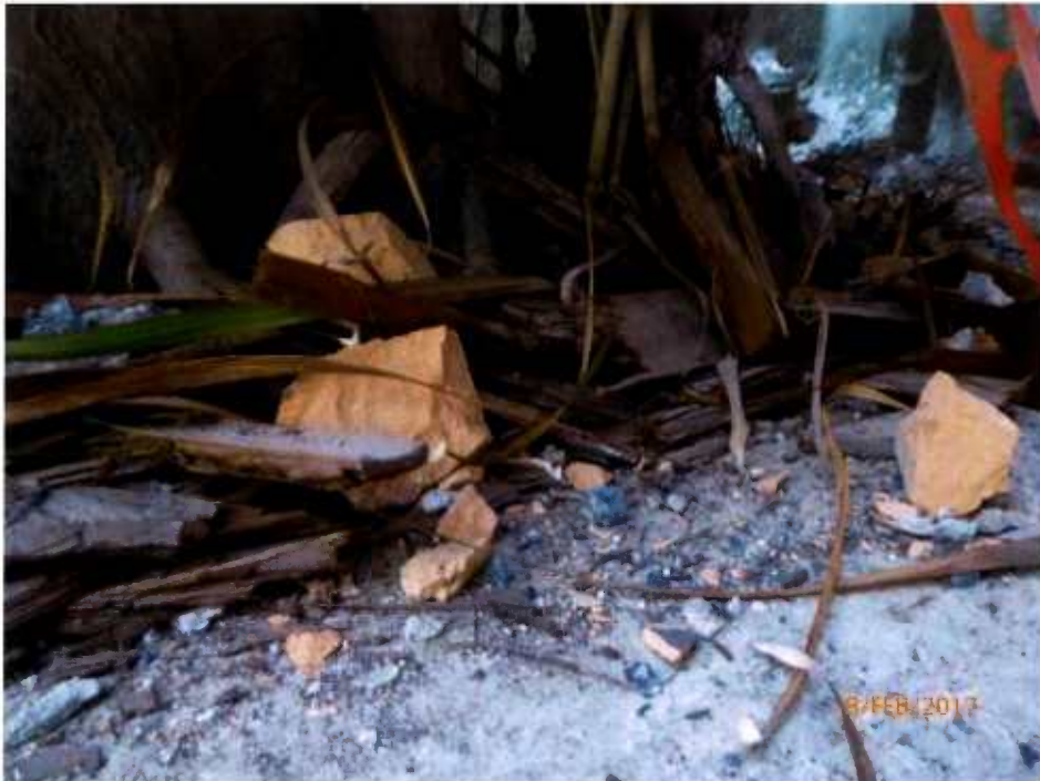
Fig. 3 A few construction debris remain at the planter.
