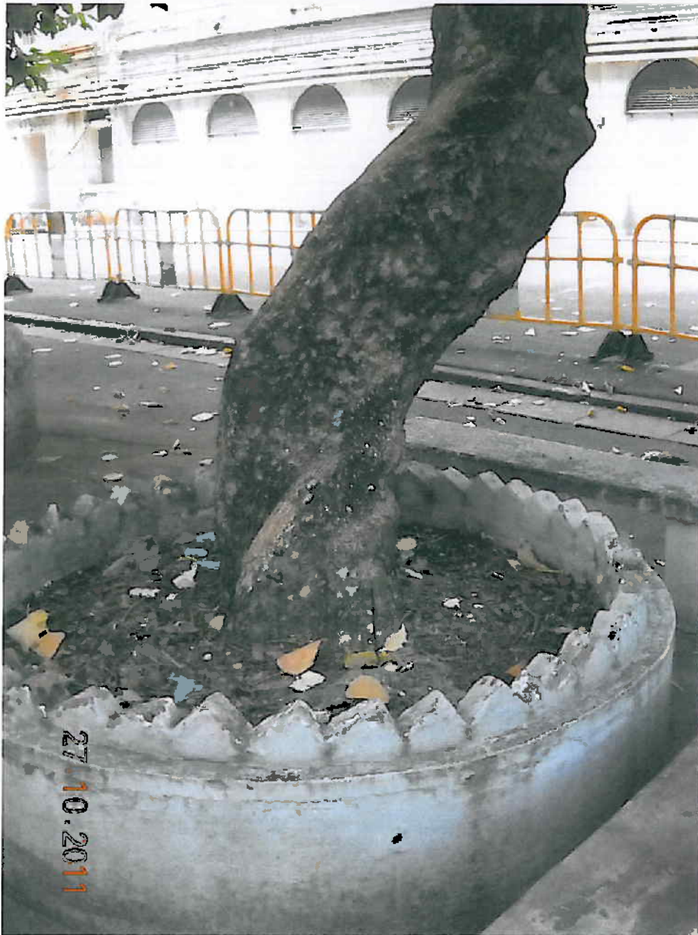
Photo 5. Condition of root flare. Tree is growing in a raised planter, rooting area was restricted
