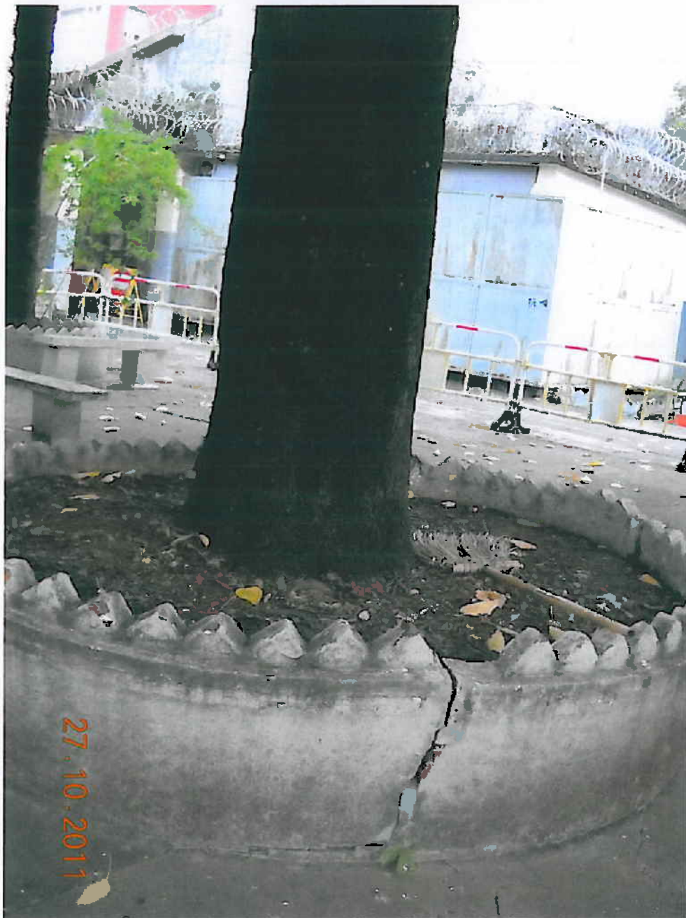
Photo 4. Condition of root flare Tree is growing in the raised planter. Root flare not visible. Rooting area are restricted by the planter.
