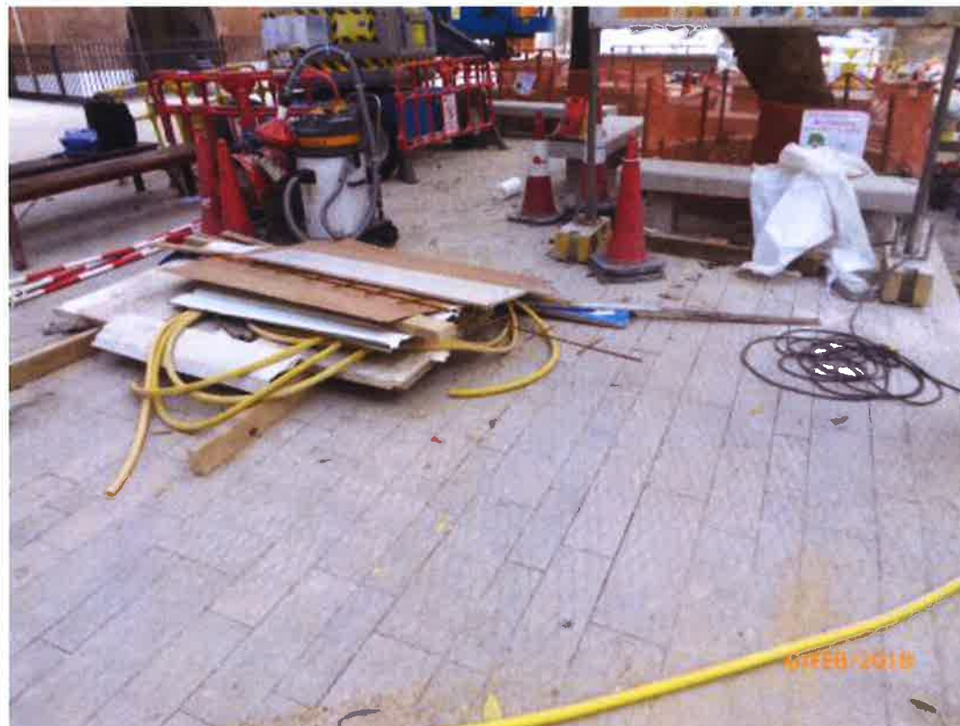
Fig. 11 Many construction materials are placed near the tree.
