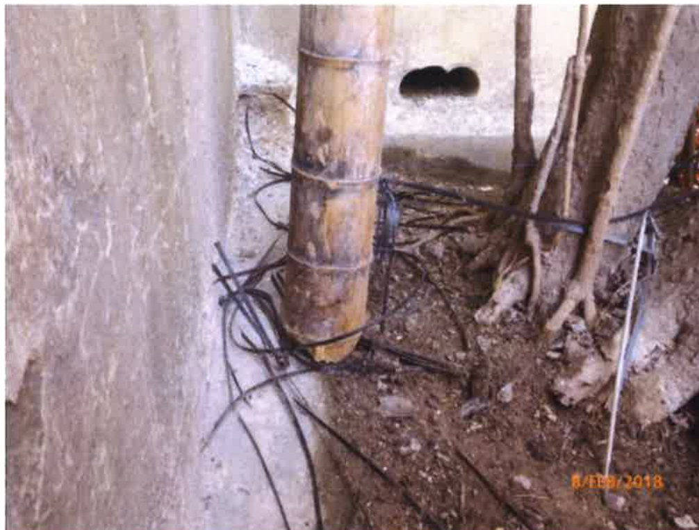
Fig. 3 A few construction debris remained at the planter.
