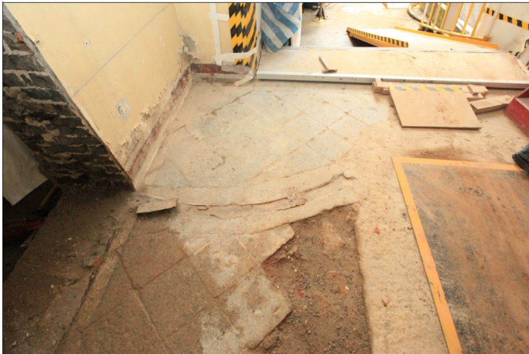
Photograph taken on 22 nd August 2013 by the Management Contractor, showing the track on the granite flagstone at the East entrance.
