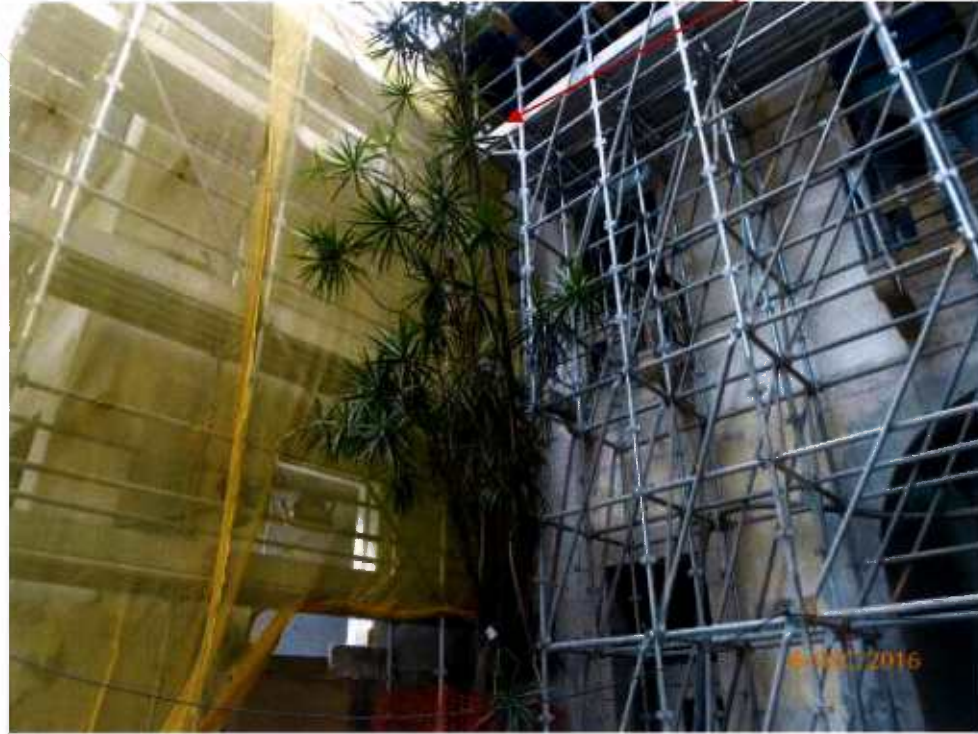
Fig. 8 Renovation works are in progress near Tree-11. We worry that these renovation works have affected the health of Tree-11 .
