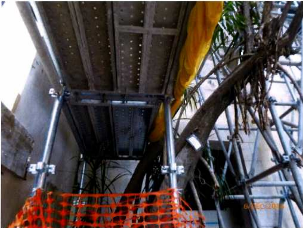
Fig. 7 A working platform is set up near Tree-11. It will affect the growth of the tree.
