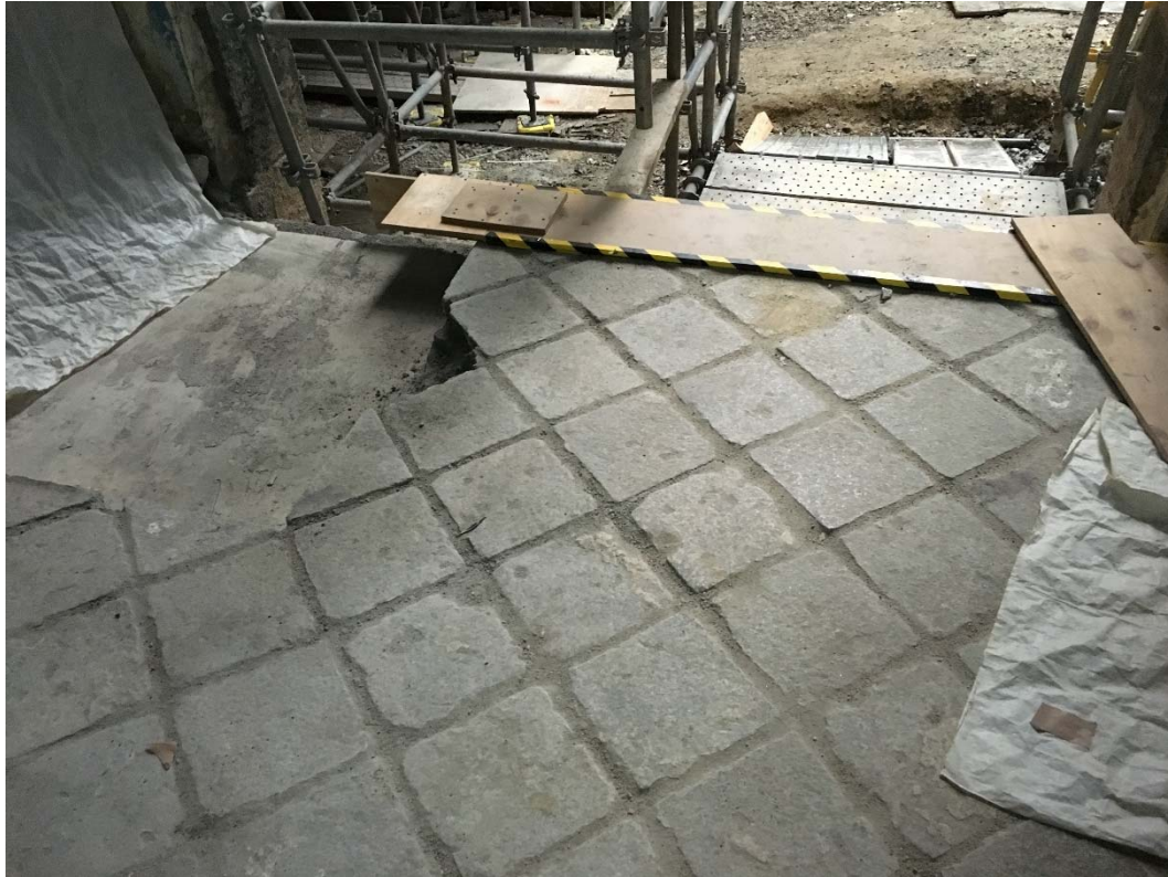
Photograph taken on 8 th November 2016, showing the incorrect granite laying
