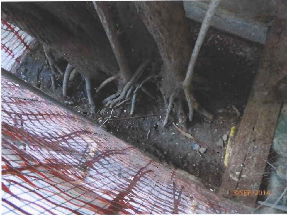
Fig. 2 The root collar is normal. The planter appears clean and tidy.
