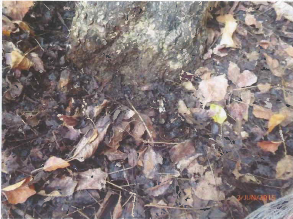
Fig 2. Root collar is normal. The planter is covered with moist mulch and fallen leaves.
