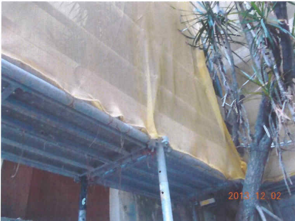
Fig. 5 The scaffold is still set up near the tree for renovation work.
