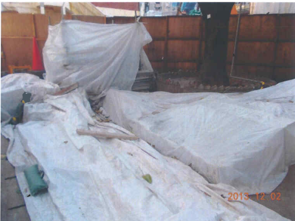
Fig. 3 Heaps of large construction materials are placed near the tree.
