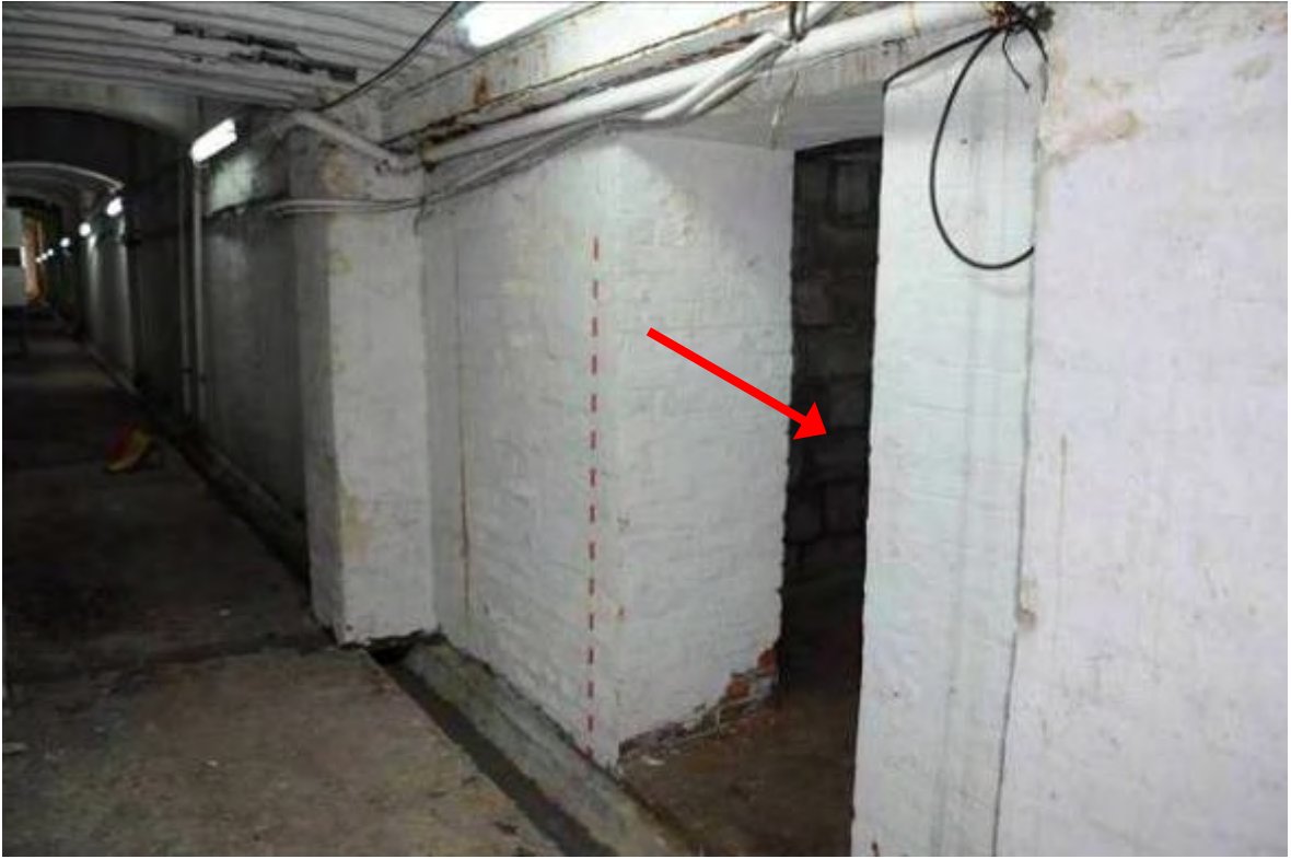
General view of the entrance to S12 inside the service corridor between the Parade Ground and Headquarter Block (view from northwest)
