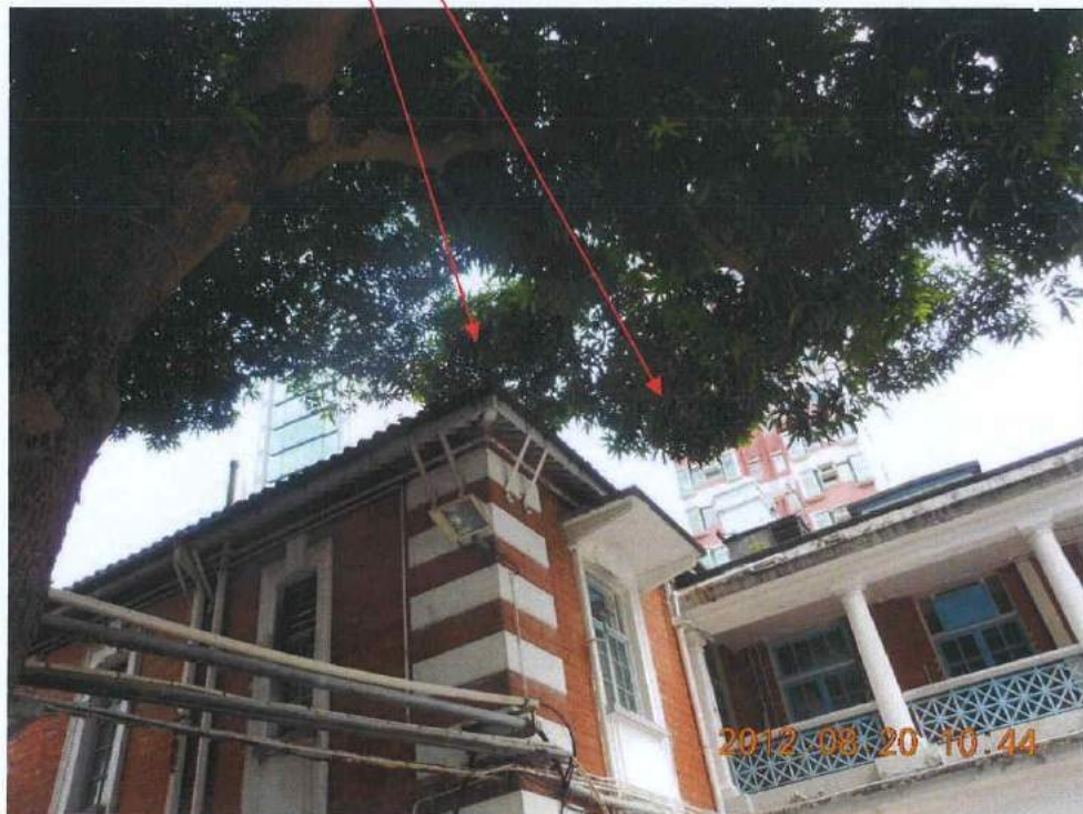
Fig. 5 Some lower leaves are too close to the nearby buildings. Trimming of such leaves is recommended..
