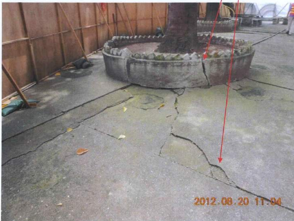
Fig. 3 The site appears clean and tidy . However, many cracks are found at the planter and the nearby ground surface.
