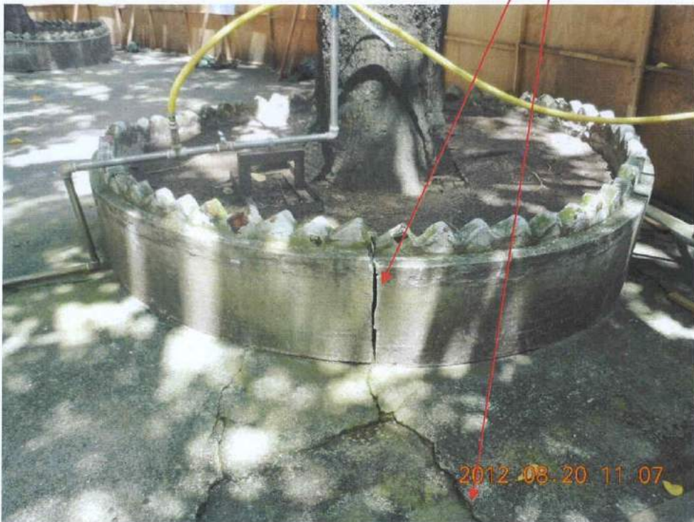
Fig. 3 The site appears clean and tidy. However, many cracks are found at the planter as well as the nearby ground surface.
