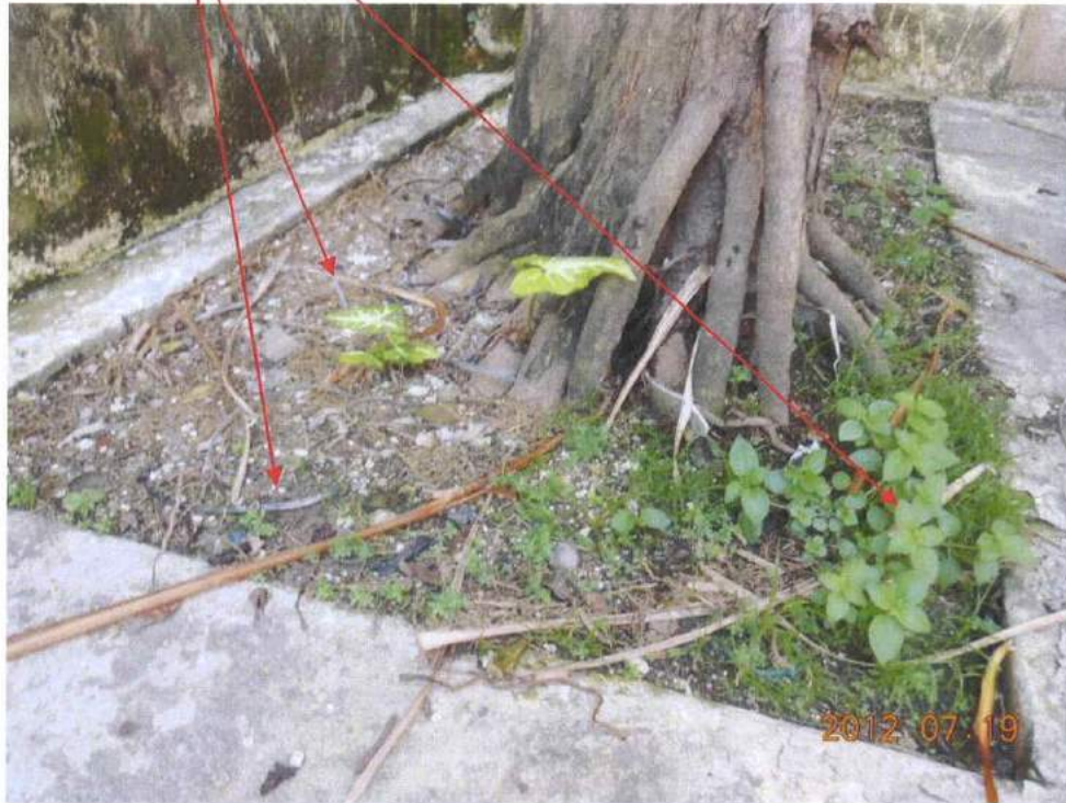
Fig. 2 Litter and weeds were found at the planter on 19 th July 2012.
