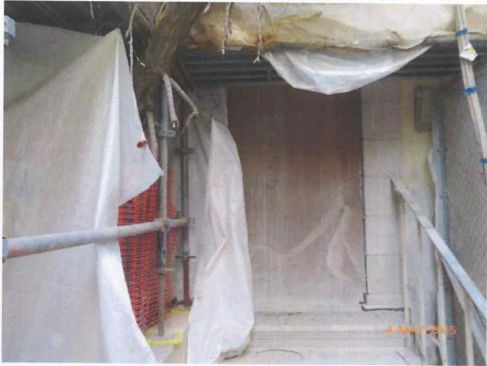
Fig. 10 The door next to Tree-11 is closed at the time of inspection.
