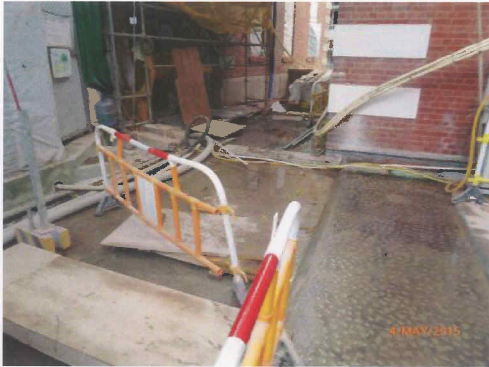
Fig. 12 Cleanliness of the site outside the cordon zone is acceptable.
