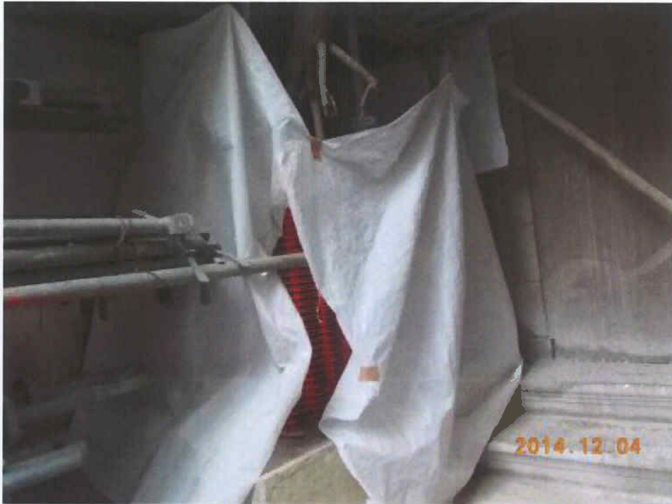
Fig. 8 A PVC cloth covers the small cordon zone to protect the tree.
