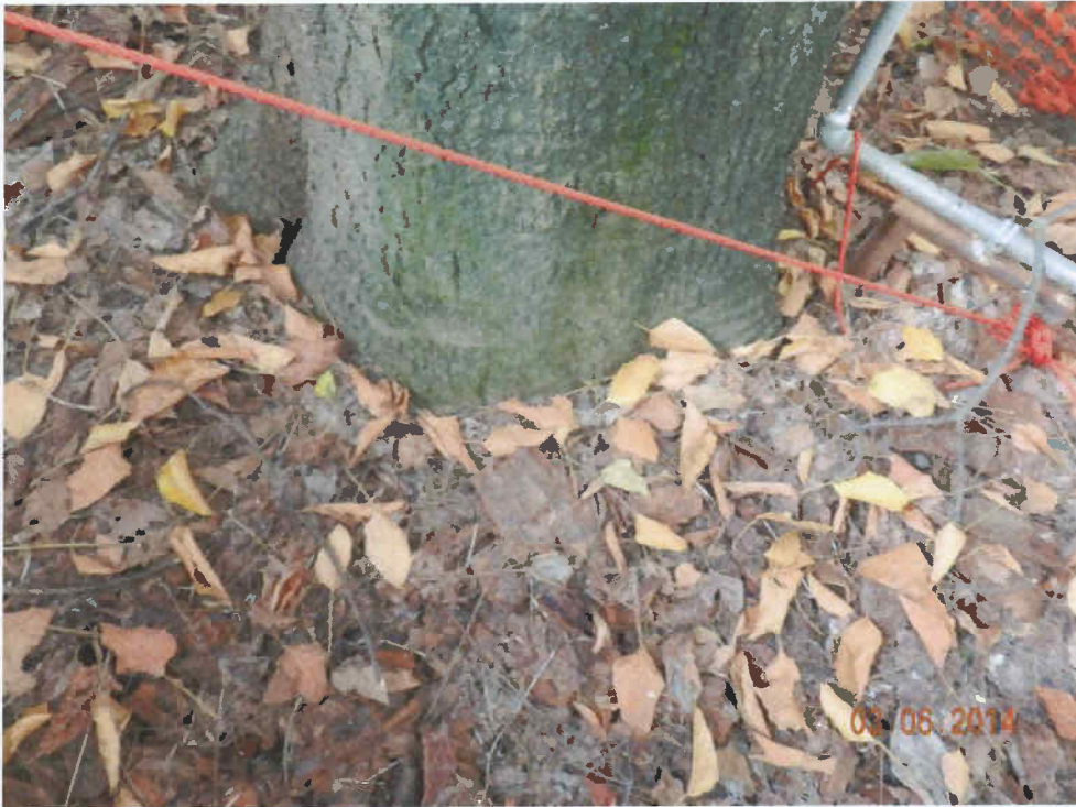
Fig 2. Root collar of Tree-7 is good. The planter is full of mulch.
