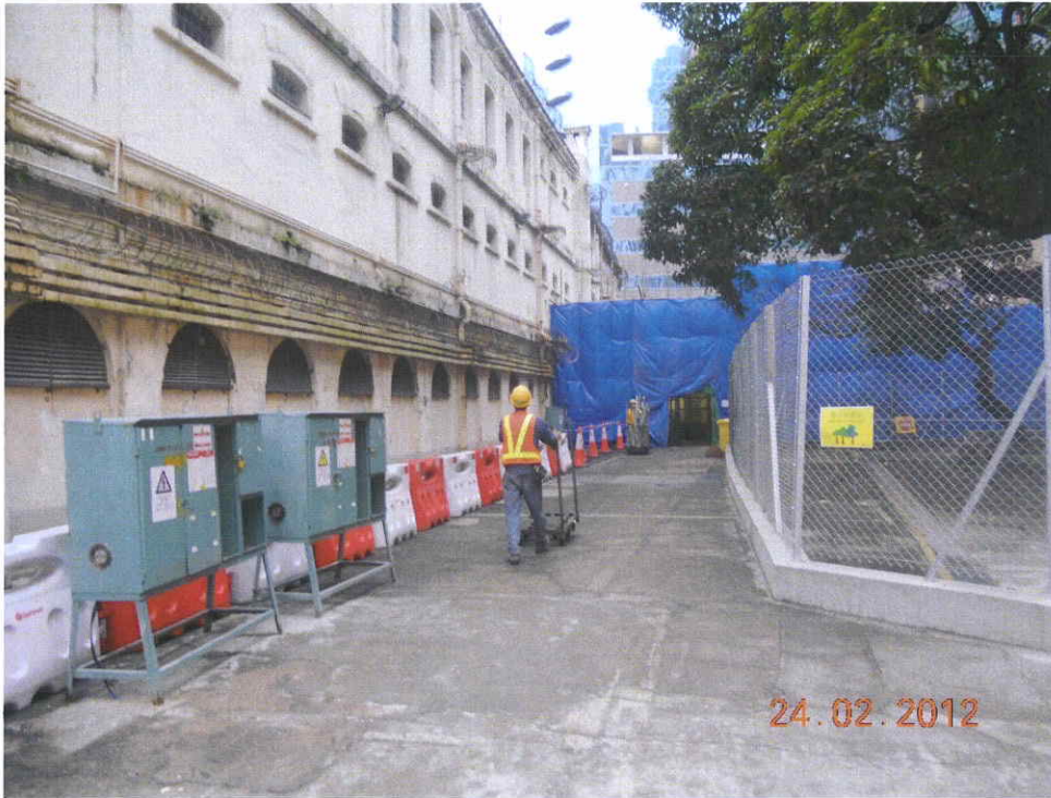
Fig. 8 The nearby area is clean and tidy. Good management on the site.
