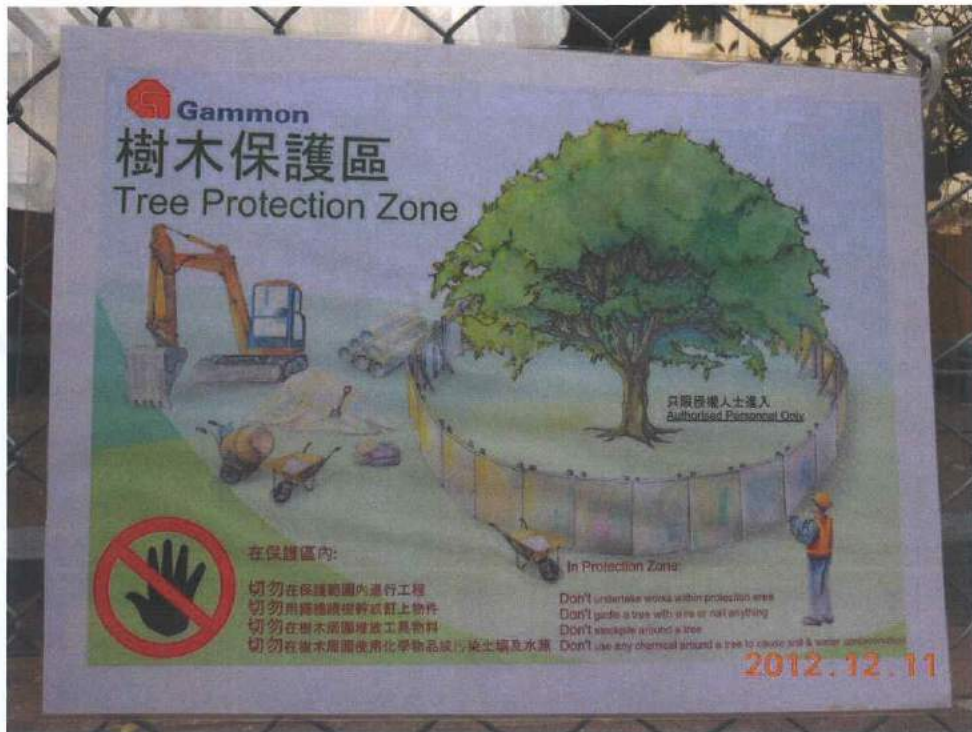
Fig. 6 Appropriate notice displays in front of the cordon zone.
