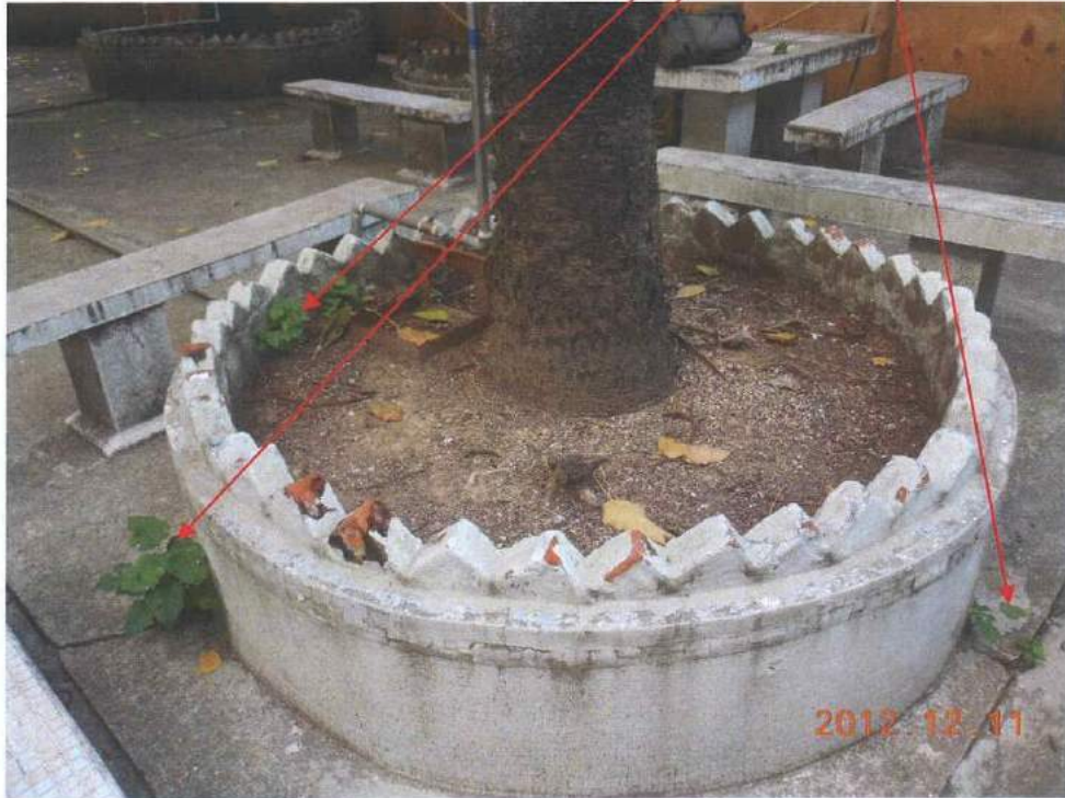
Fig 2. Cleanliness of the planter is acceptable. The undergrowth near Tree-9 should be removed.
