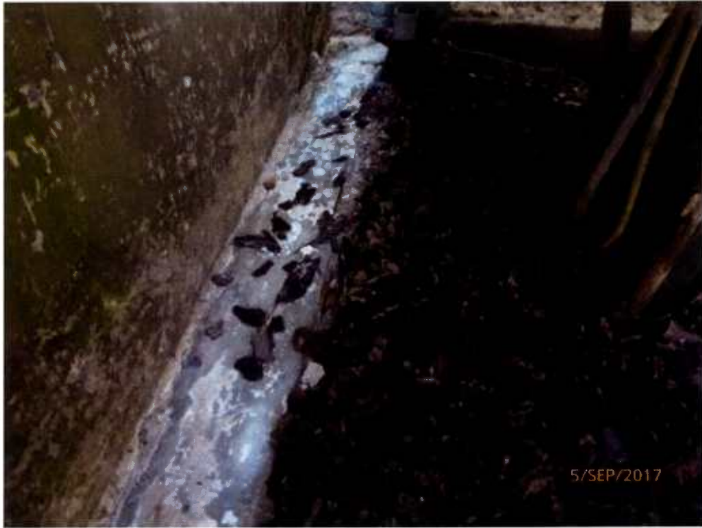
Fig. 4 Construction debris had been removed away prior to inspection on 5 th Sept. 2017.
